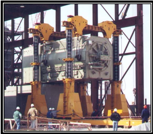
J&R 1402-4-39 Octagon LIFT-N-LOCK Hydraulic Boom Gantry with 150 Ton PowerLinks on a project in Riyadh, Saudia Arabia
